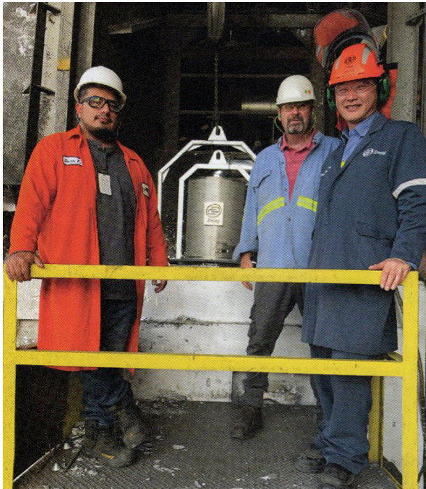
Figure 2. Standing in front of the MagPump installed in the pump well of the furnace (L-R): Oscar Perez, plant manager for TST's Fontana operation; Tom Moore, aluminum casthouse sales engineer, The Schaefer Group, Inc.; and Eishin Takahashi, president of Zmag America.
