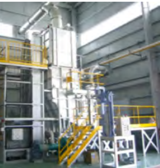
Tower or Stack Melter
